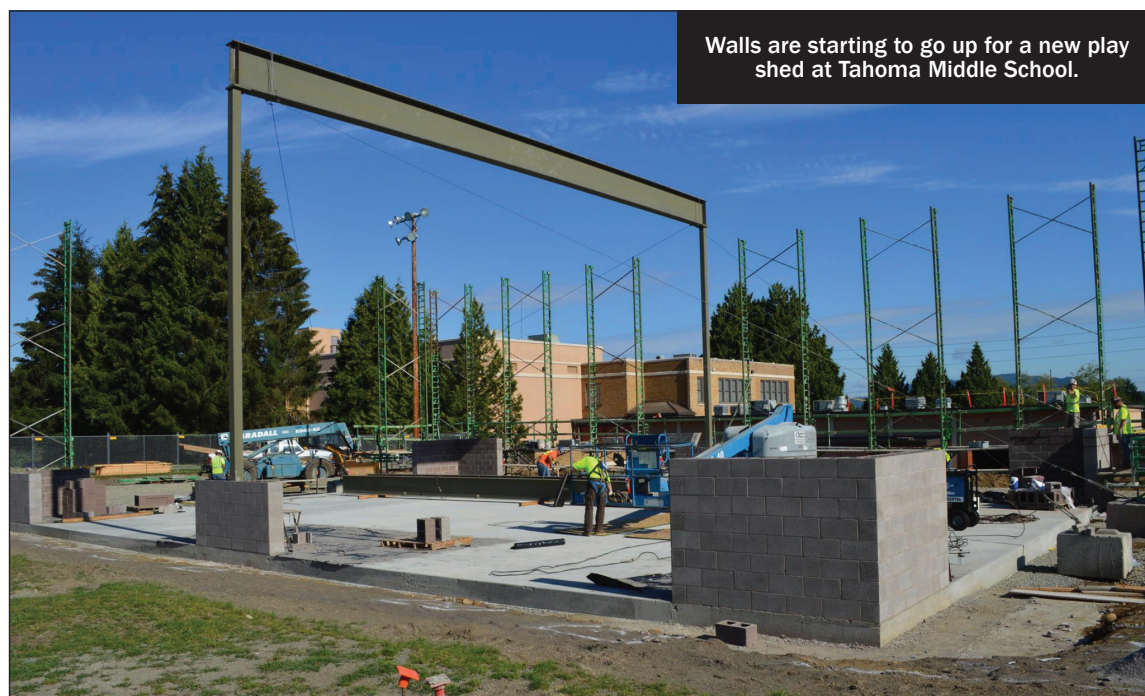
Cedar River Middle School is being converted to an elementary. The work shown here is for the main entrance.
