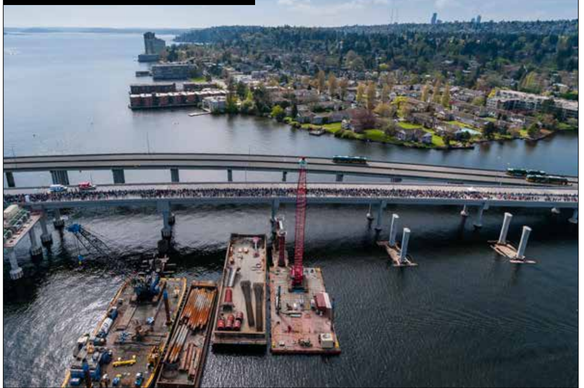
Crews from Flatiron West are working on the West Approach Bridge North project.
